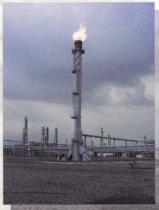
Petrochemical Plants, Refineries, Metering Stations
